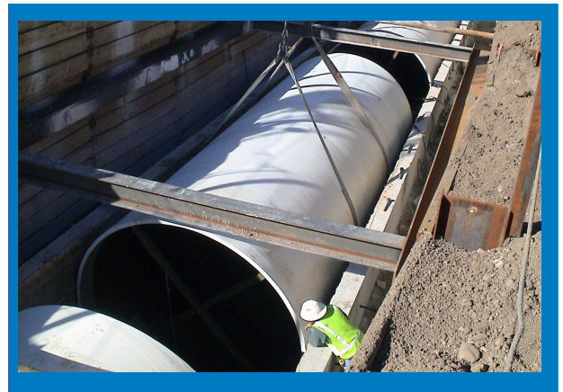
The 28-foot pipe sections were lowered through a 29-foot wide "window" then rolled into place.
