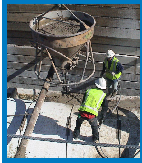
Concrete grout was poured in the space between the pipe and trench wall.
