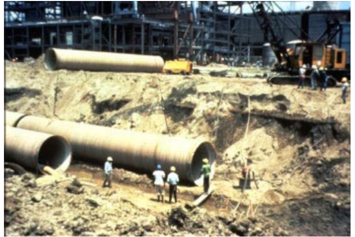
The light weight of the composite versus steel facilitated installation. Composite components in underground and aboveground sections are in very good condition after decades of use.
